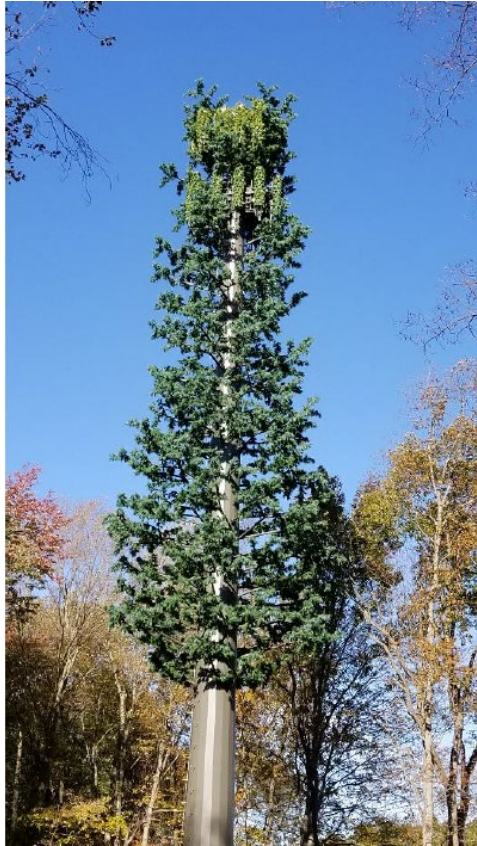
Example of a 120-ft tall Homeland Tower stealth tree monopole design.
