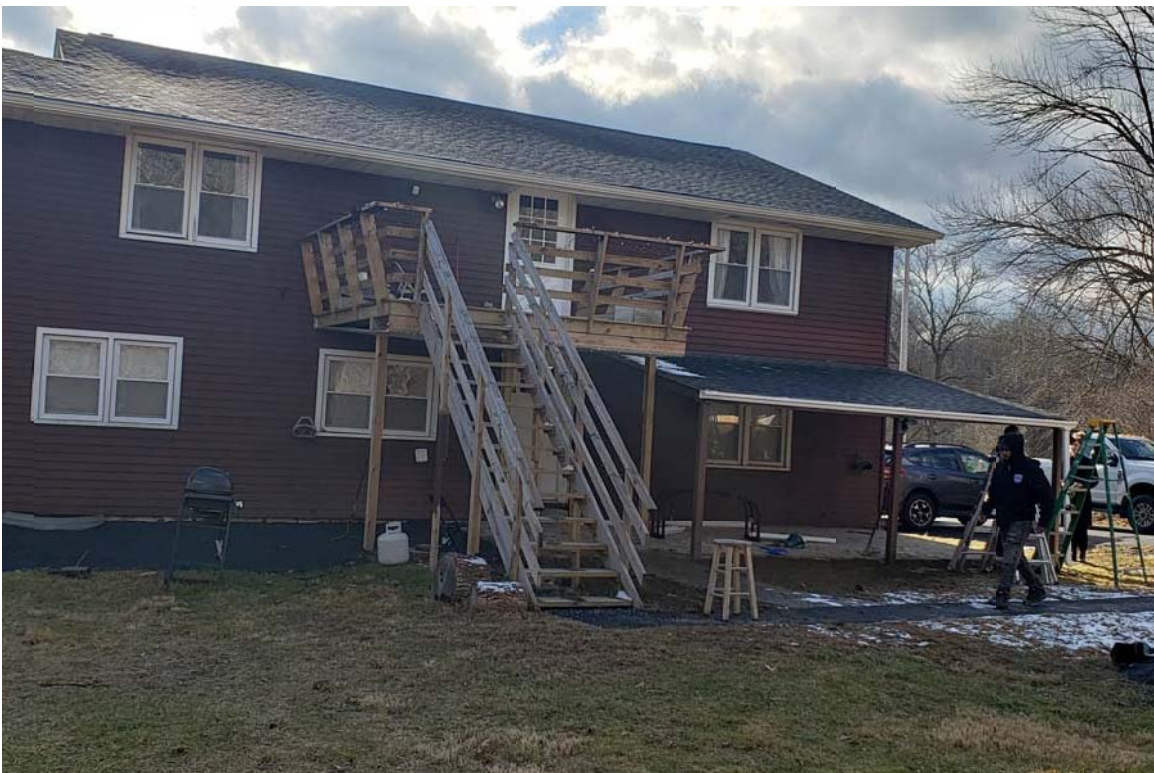
FIGURE 8: NORTH SIDE OF RESIDENCE, DECK ACCESS TO SECOND STORY & NORTH ACCESS TO GROUND FLOOR UNIT
