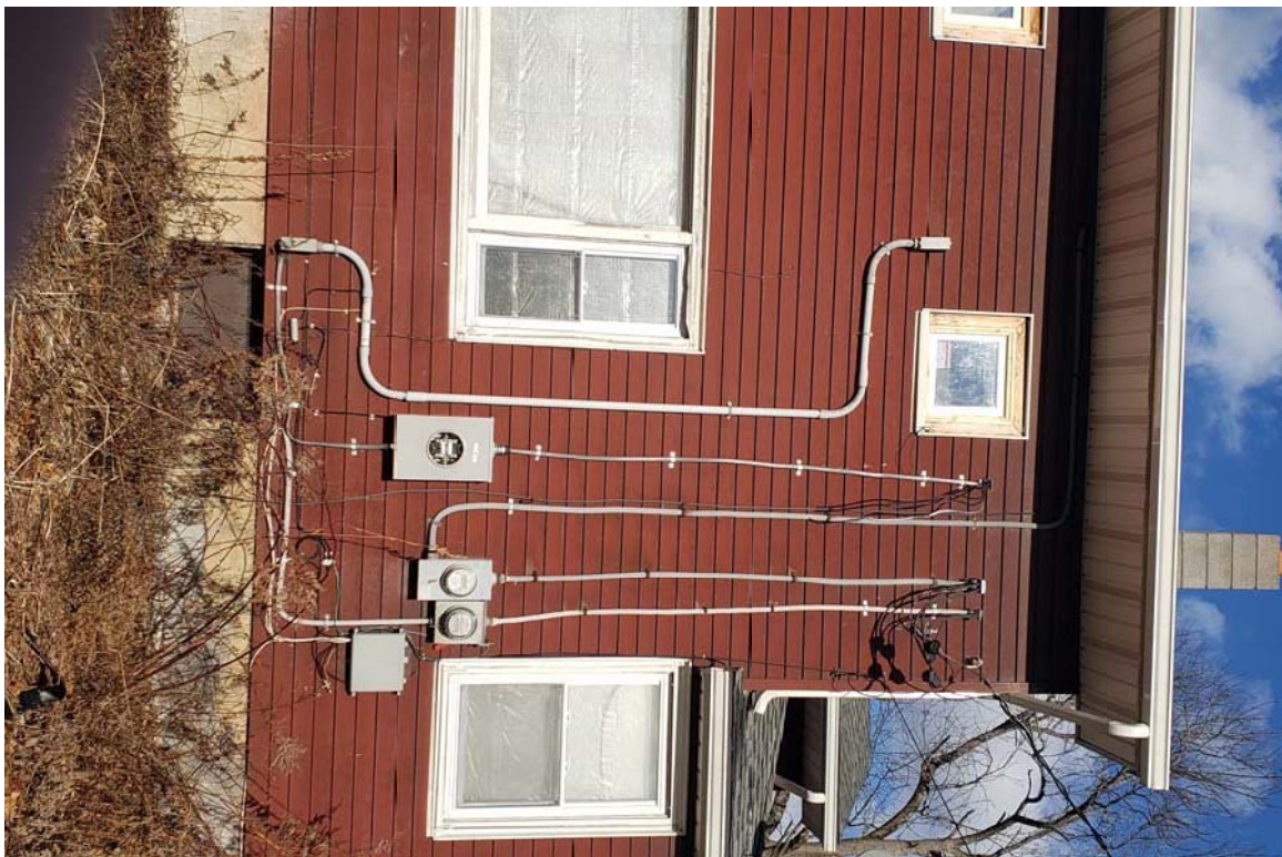
FIGURE 6: SOUTH SIDE OF STRUCTURE - ELECTRIC METERS (LEFT IS SERVICING UPPER UNIT, RIGHT IS SERVICING LOWER UNIT)
