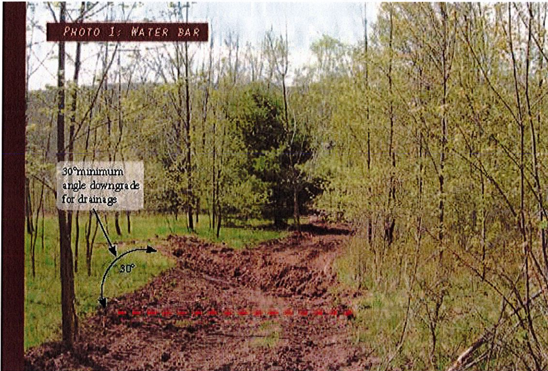
Waterbar in skid trail
