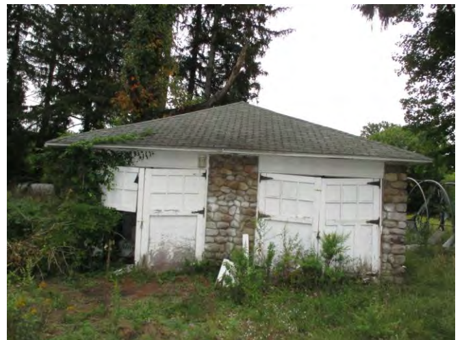
Photo 12 General View of Dilapidated Garage
