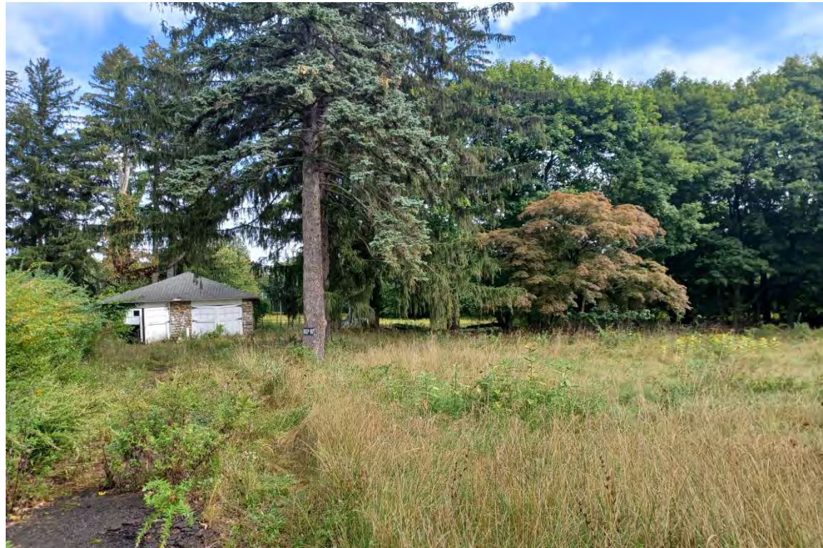
Photo 4: A dilapidated garage and Quonset hut are located to the northeast of the residence. The asphalt driveway leading to the garage is overgrown. View to the northeast.
