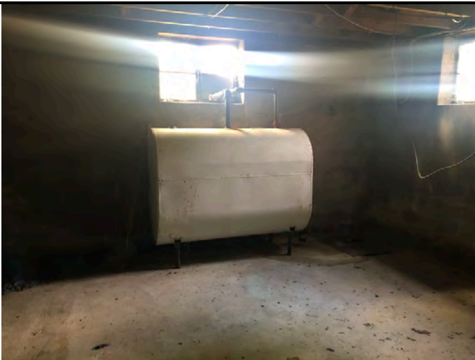
Site Building 1 275 gallon fuel oil AST
