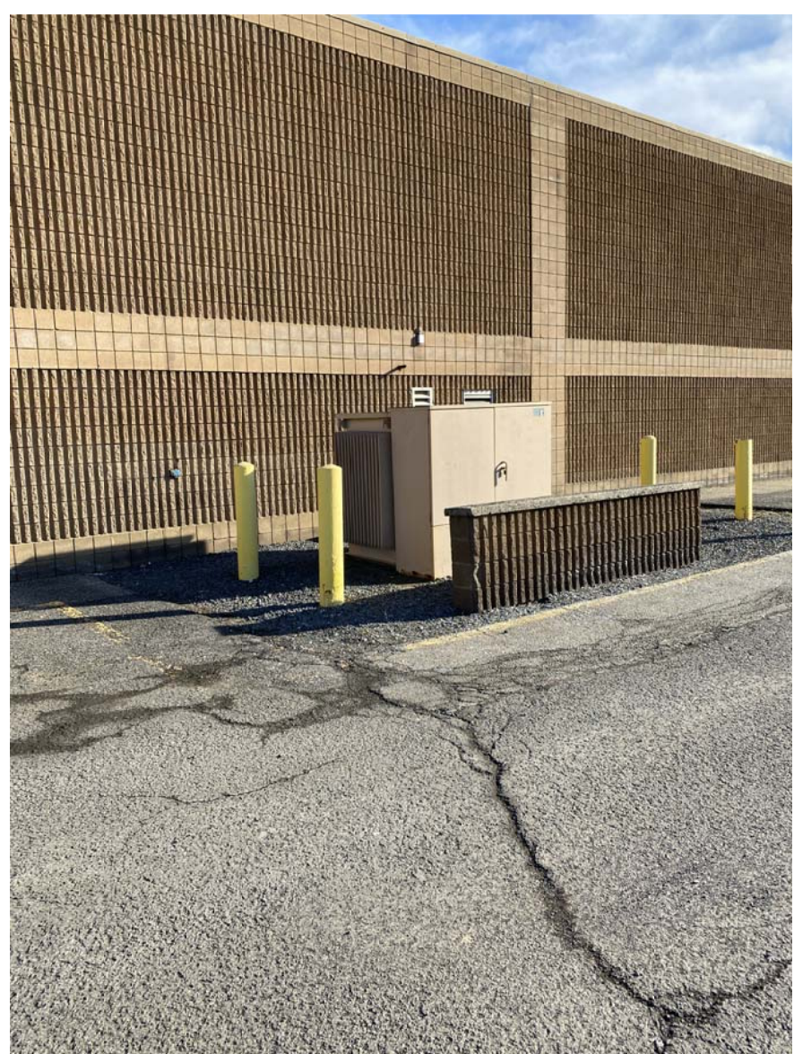
③ EXISTING TRANSFORMER
