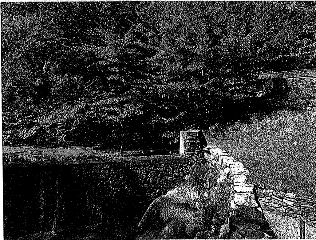
VIEW LOOKING AT THE BACKSIDE OF THE EMBANKMENT FROM ACROSS THE DAM
