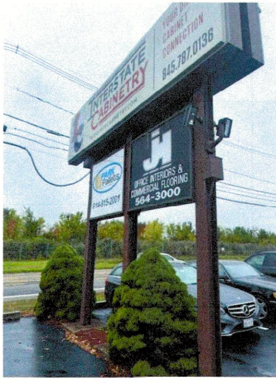
EXISTING EXTERIOR LIGHTS ON EXISTING SIGN
