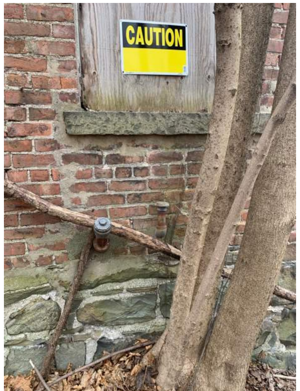
Fuel Tank Vent and Fill Piping on East Side of House
