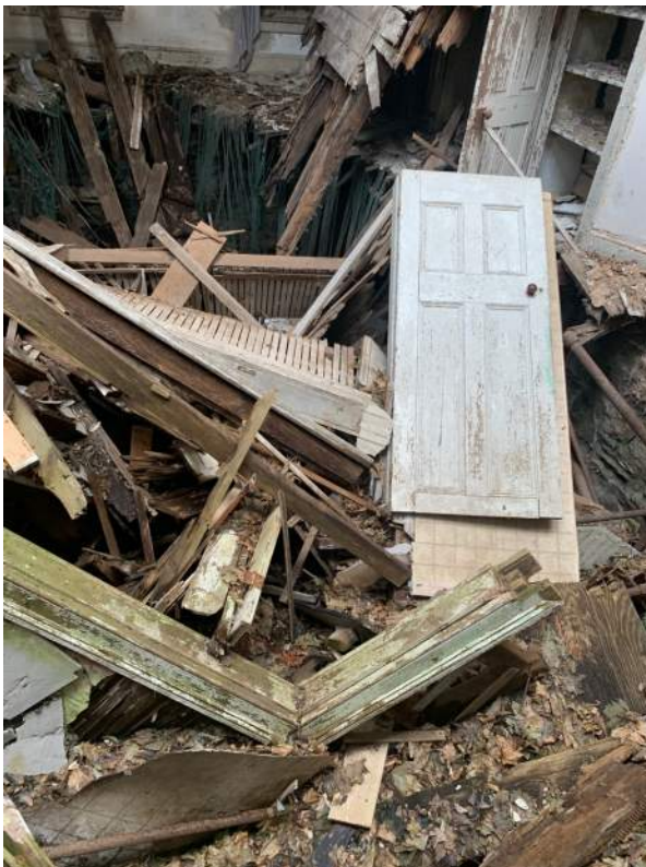
Collapsed floor area inside house from south window
