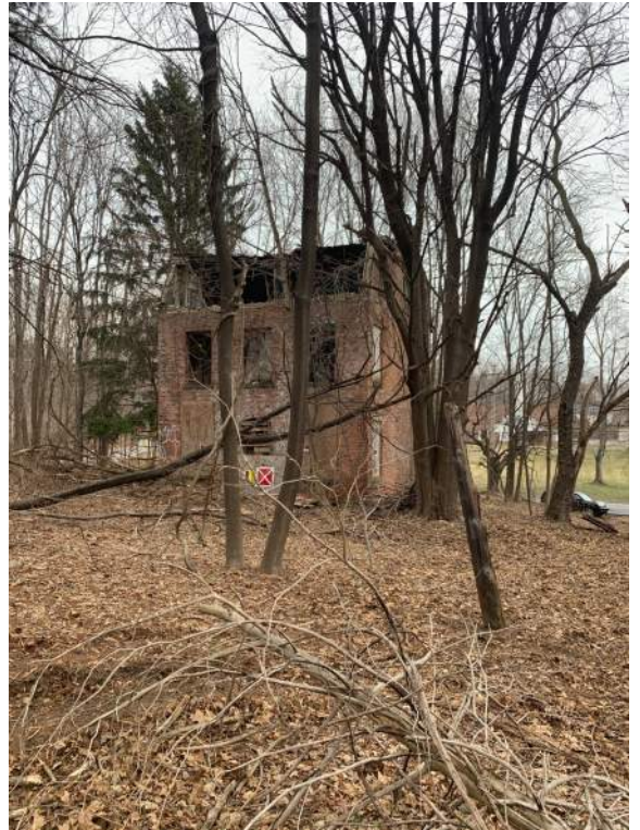
Site House South Side – Note collapsed roof area
