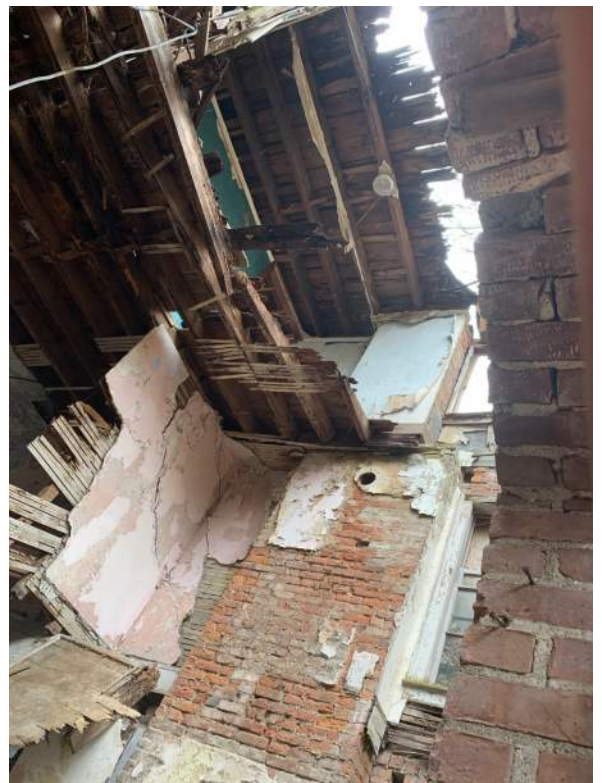
Collapsed house roof interior Area from south window
